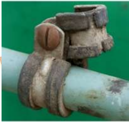
Fig. 1. Vibration-induced failures in hydraulic pipelines [28].
