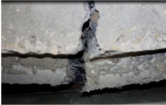
Fig. 12. Expanding the crack and increasing the crack width and bridging action of the fibers in specimen RSWH3PN2G6x2
