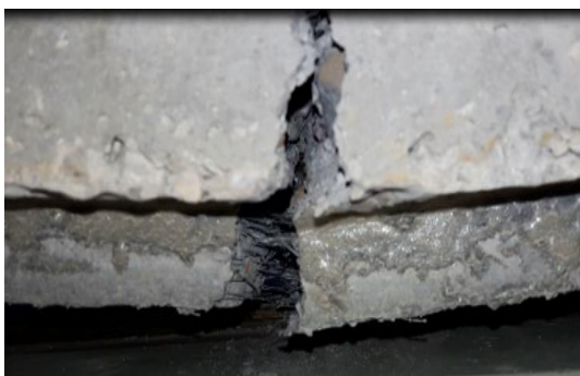
Fig. 14. Expanding the crack and increasing the crack width and bridging action of the fibers in specimen RSWH3PN6G2x2
