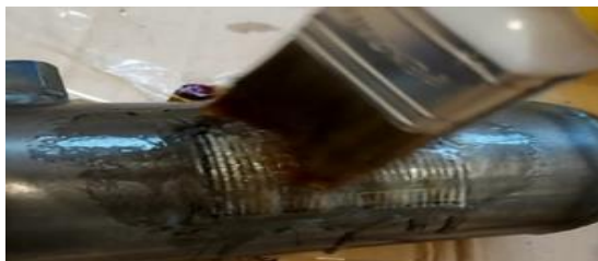
Fig. 2. Repair of cracked steel pipe using composite patches by the hand lay-up method
